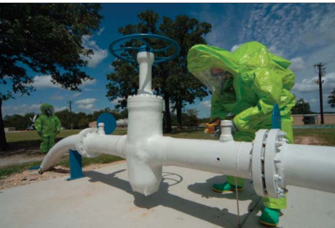
TEEX has completed a 2,300-ft belowground pipeline with multiple aboveground connections to train emergency responders to manage and mitigate pipeline emergencies. The project, which can leak both liquid and gas, was constructed with input from the world's leading pipeline industry representatives.
