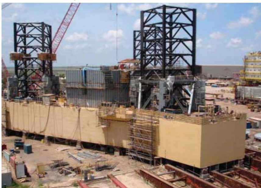
One of five Scorpion Offshore Jackups under construction, the Scorpion Courageous will be delivered in 2007.
